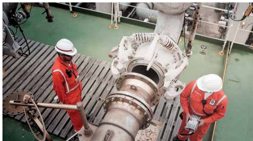
FIG. 3. Maintaining the safety of personnel and property was the highest priority of the Qatargas JBOG project.
