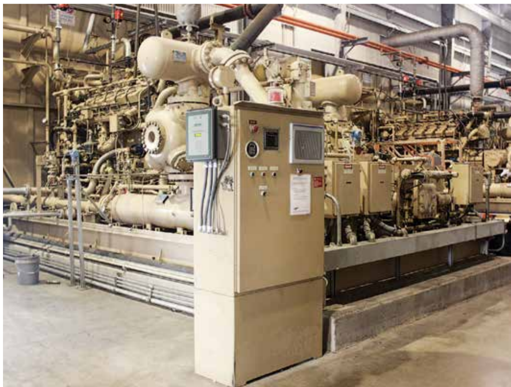
FIG. 1. Each compression station, located at 40-mi to 100-mi intervals along the pipeline route, utilizes two to 10 compressors in the 2,000-hp (1.5-MW) range.
