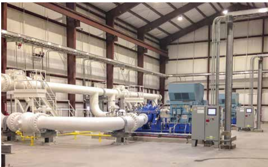
FIG. 1. The conversion of an existing gas pipeline into a crude oil pipeline required the installation of new equipment at a series of pumping stations.
