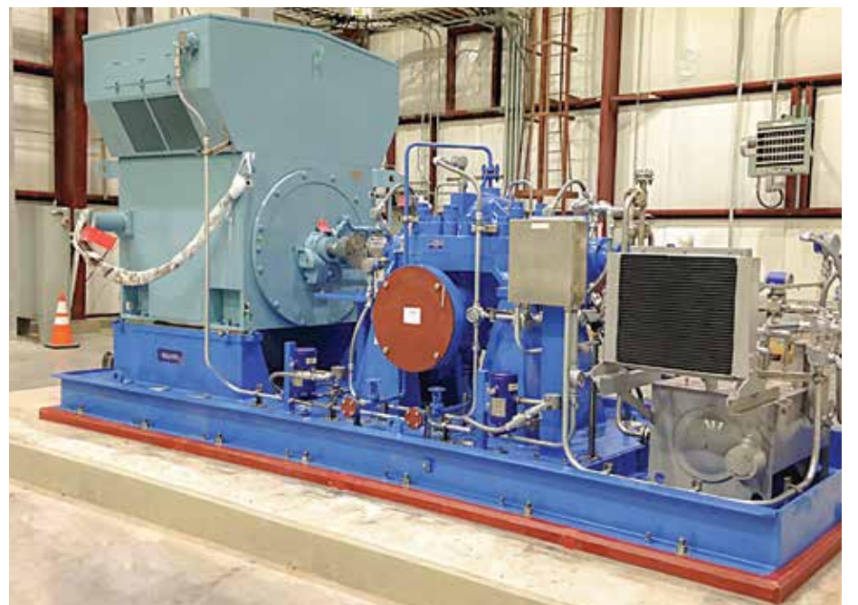
FIG. 3. The Sulzer pump skids were designed to typical pipeline configurations, but tailored to the customer's specific requirements.
